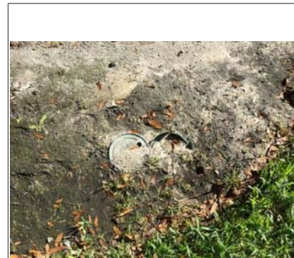
Damage irrigation valve box in rear planter bed
