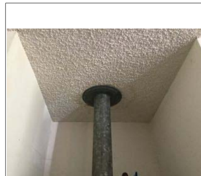
Moisture staining around water heater vent pipe ceiling penetration
