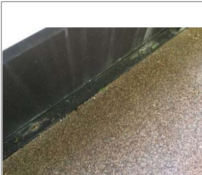
Screen enclosure anchor bolts beginning to rust / anchor bolts missing / loose screen panel(s)
