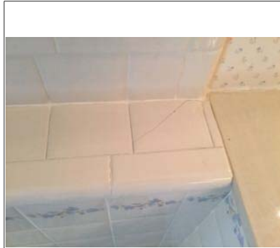
Cracked tile along tub shelf
