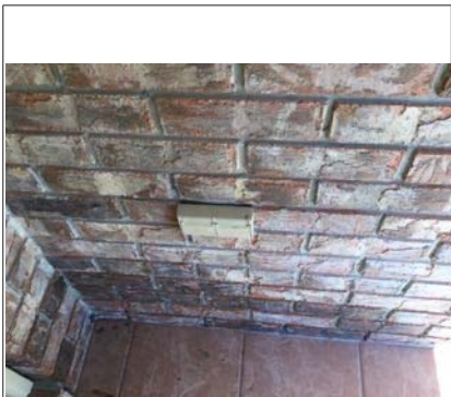
Loose electric outlet on front porch
