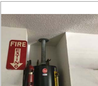
No combustion air vent present for gas water heater
