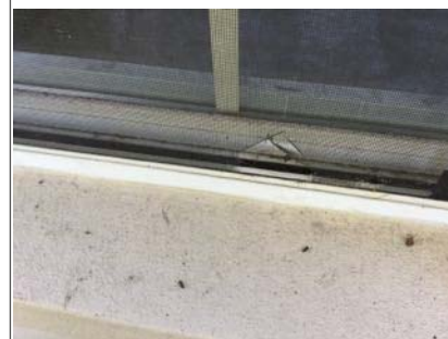
Torn / worn window screen(s) present
