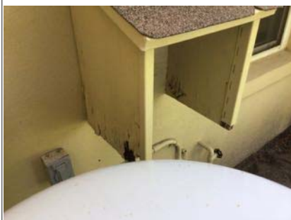
Moisture damaged wall box behind well equipment
