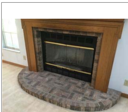
Recommend performing annual flue maintenance prior to use
