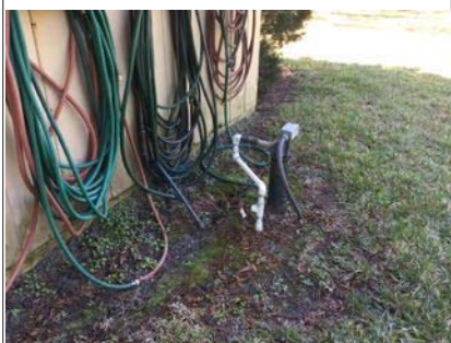
Well head exposed to elements
