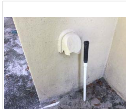
Chimney vent cover brittle / cracking
