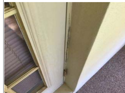
Caulk / Paint beginning to flake around bathroom door
