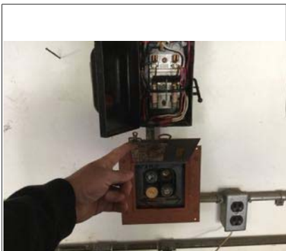
Fused electric circuits present in garage , recommend electrician evaluate
