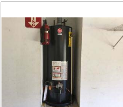
Gas water heater 5 years old
