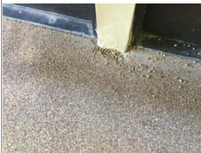
Rear lanai floor finish beginning to flake around base of post
