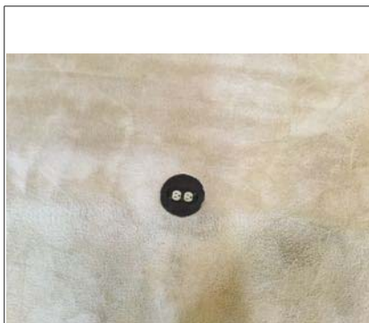
Floor outlet missing cover
