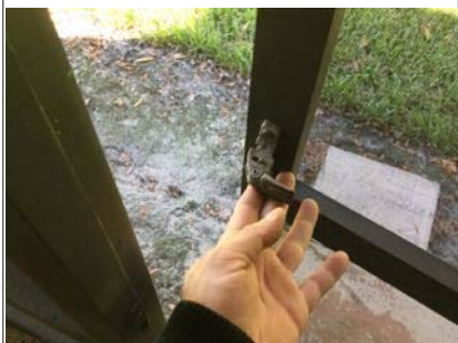
Rear enclosure door hardware not operating properly
