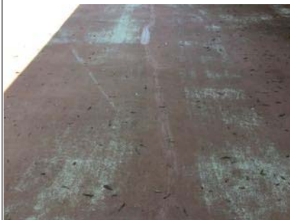
Typical concrete cracking through driveway
