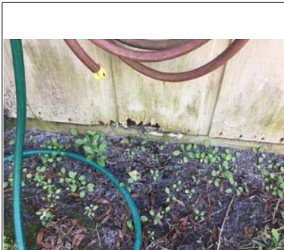
Moisture stained and or damaged siding along sill of yard shed
