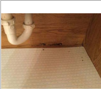
Some apparent moisture damage along bottom of vanity cabinet in master bedroom
